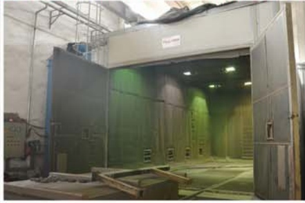
喷砂房 sandblasting room
